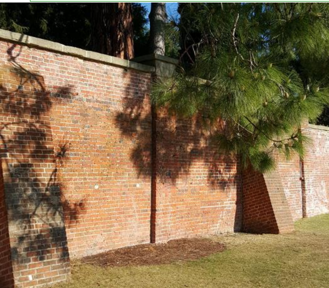
Left: Merely one section of the Arthur Wall today at the Royal Tasmanian Botanical Gardens showing the use of buttresses for strength and support. Source: gardens.rtbg.tas.gov.au
